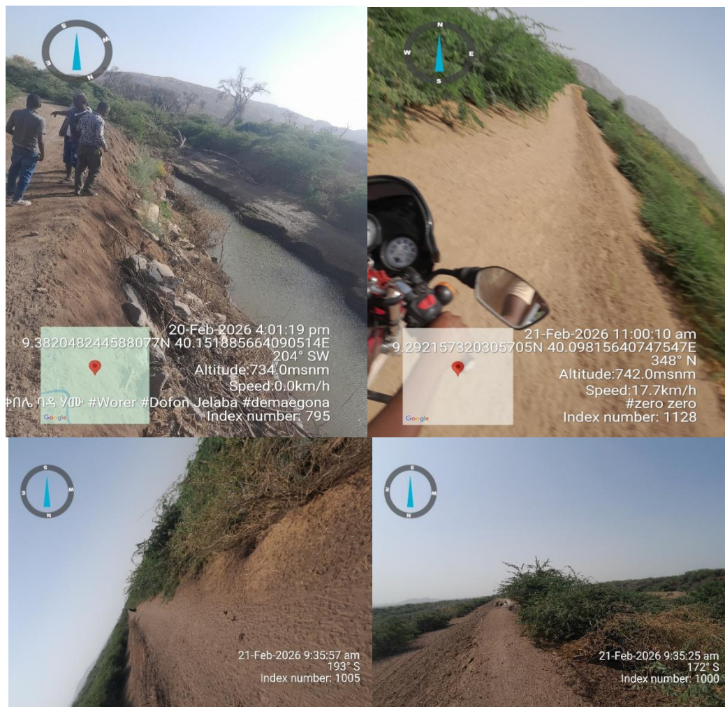
Figure 2.3: Observed threats to dike integrity: (a) Bank erosion triggered by shifting river dynamics; (b) View of the narrowed crest, slope side and dense Prosopis juliflora
